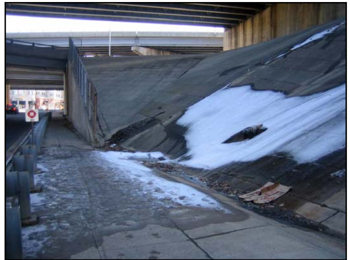
Poor drainage under I-395 overpass
